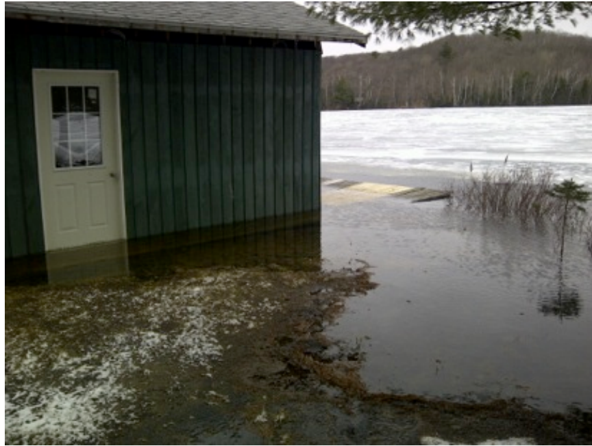
Spruce Lake Boathouse – showing overbank flooding of shoreline structure with ice still on the lake.
