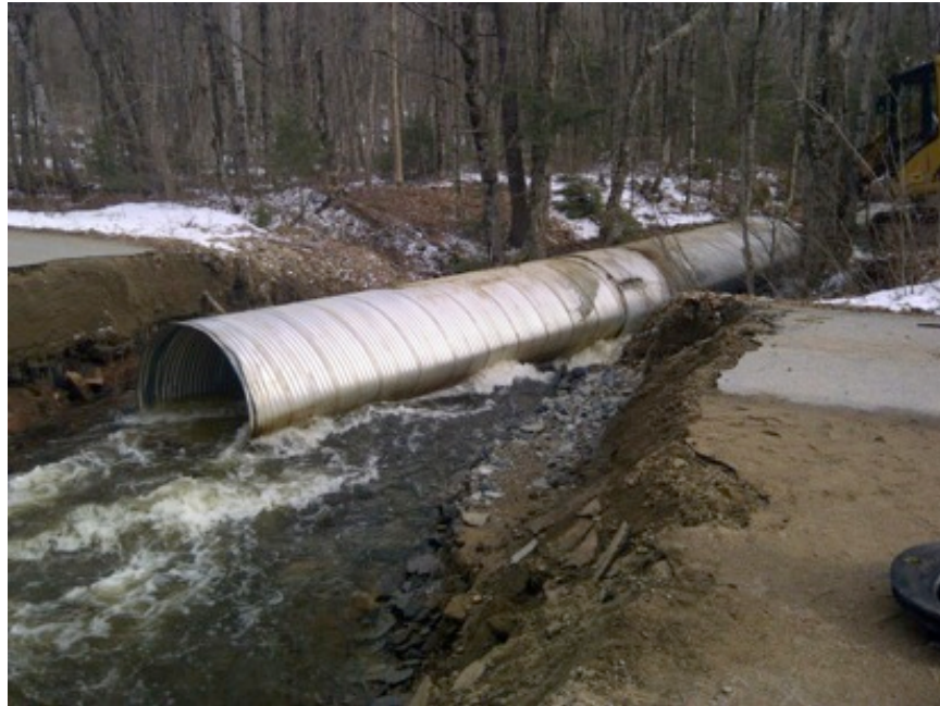
Road washout on route to Haliburton Lake
