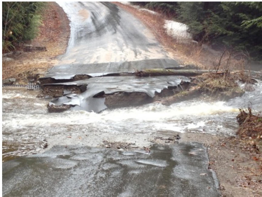
Wilkinson Road, Kennisis Lake washout of culvert
